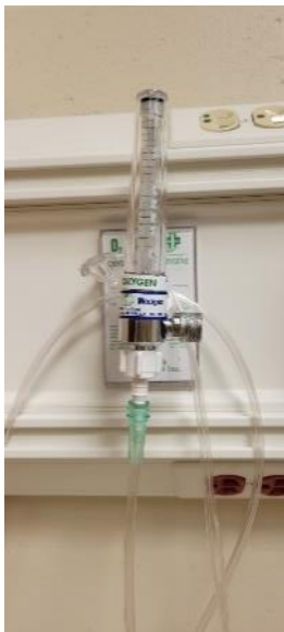
Wall Mounted Oxygen Regulator (functioning)
